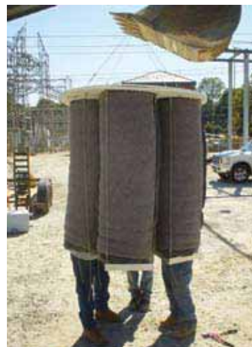
Catch basin drain filters.
